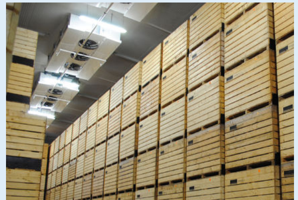
Arrangement of boxes in carrot store Green-grow, DGN aircoolers mounted in the middle
